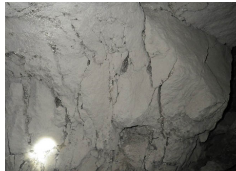
Figure 7—Photo of pillar B showing intense fracturing
