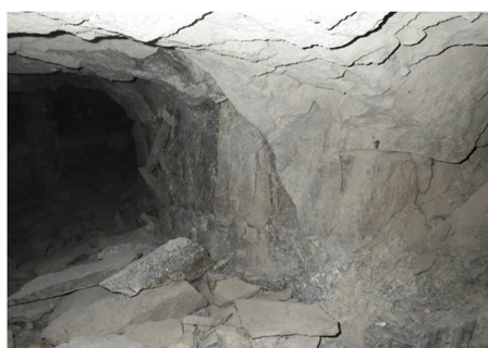
Figure 10—Photo of pillar G showing scaling
