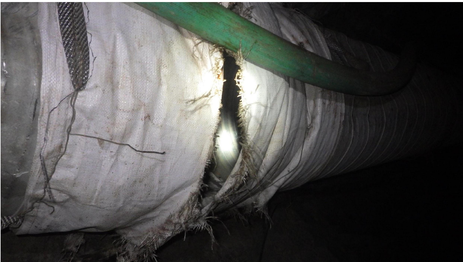
Figure A: Broken ventilation ducting
