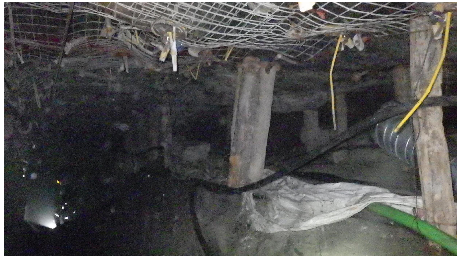
Figure B: Lack of brattices in a centre gulley
