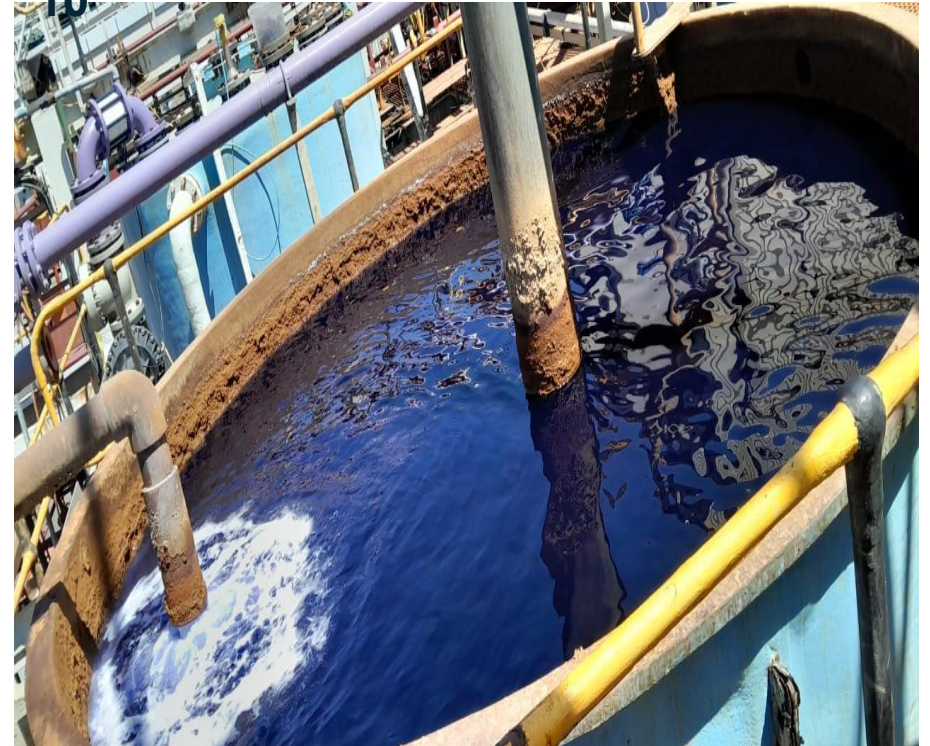
Thickener After dosing Magnafloc™ 10.
