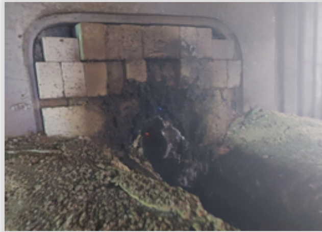
Figure 2: Smelting furnace's worn-out taphole.
