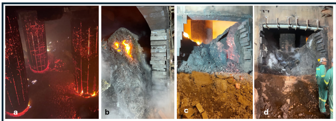
Figure 9: (a) Furnace melt down; (b) banks in front of sidewall brickwork; (c) mix, banks and chrome to be broken out; (d) steel support to prevent freeboard brickwork collapse.
