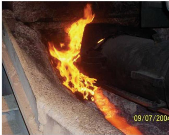
Figure 17. Excessive tap-hole clay bypass [BM7].
