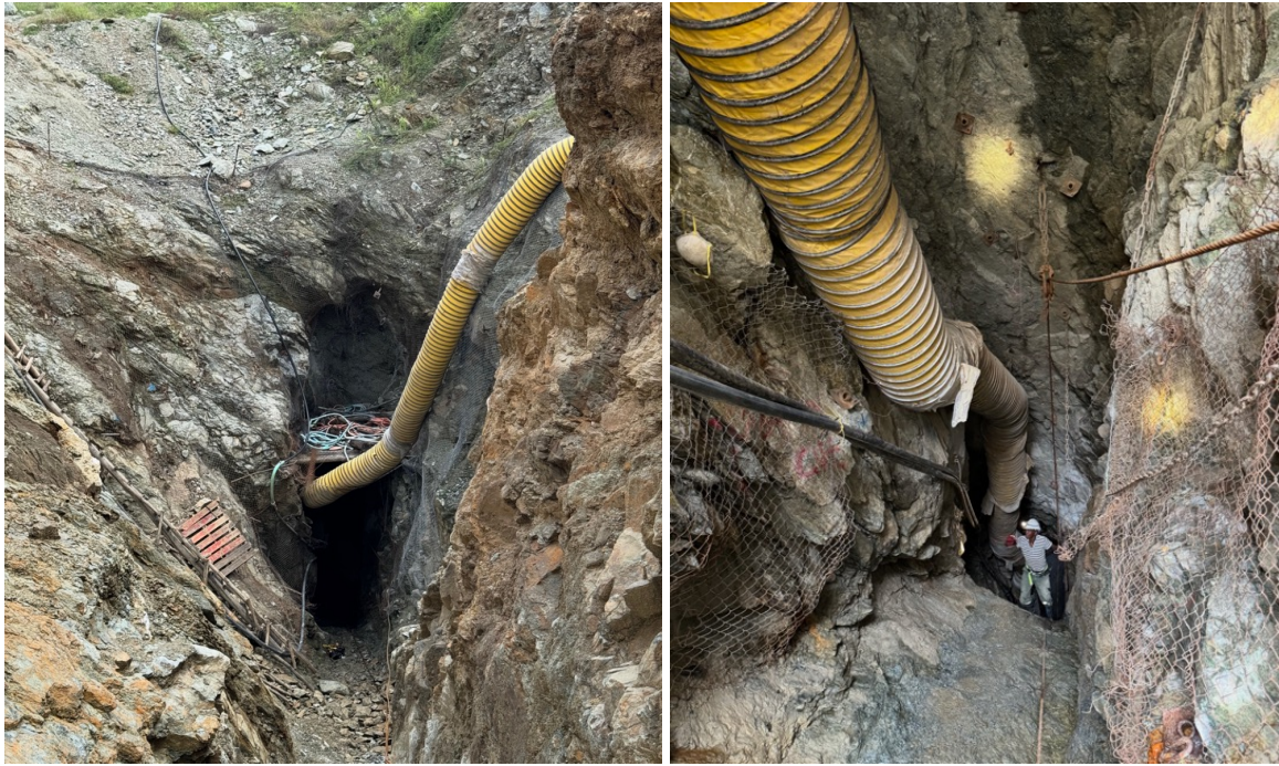
Figure 4: Ventilation in winze
