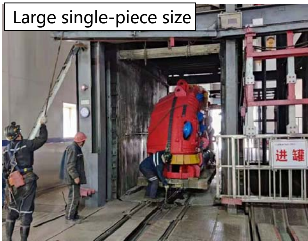
Large assembly chamber
