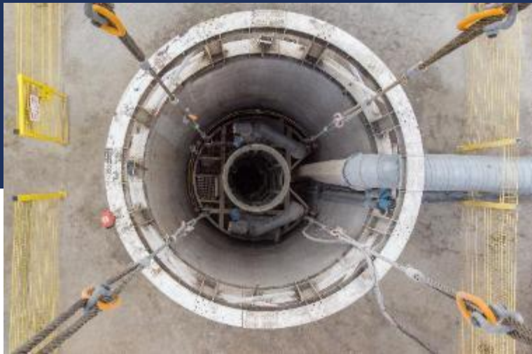
Image: The top of the SBS during testing.
