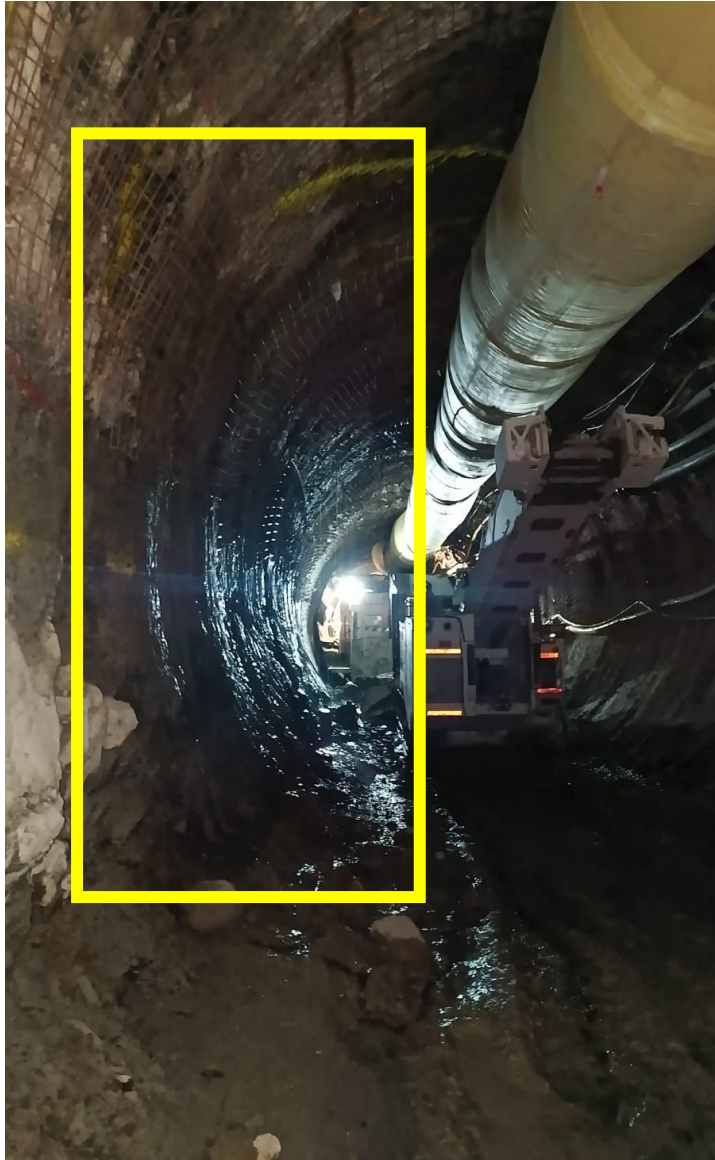
Image 25 & 26: Underground water encountered
