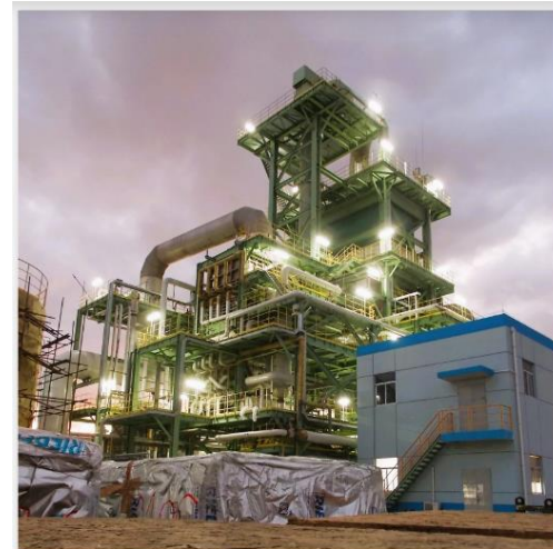
Sulfur Oxidation Plant
