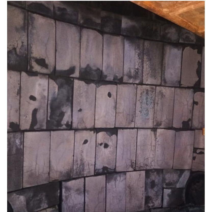
Scrubber bricks spalling
