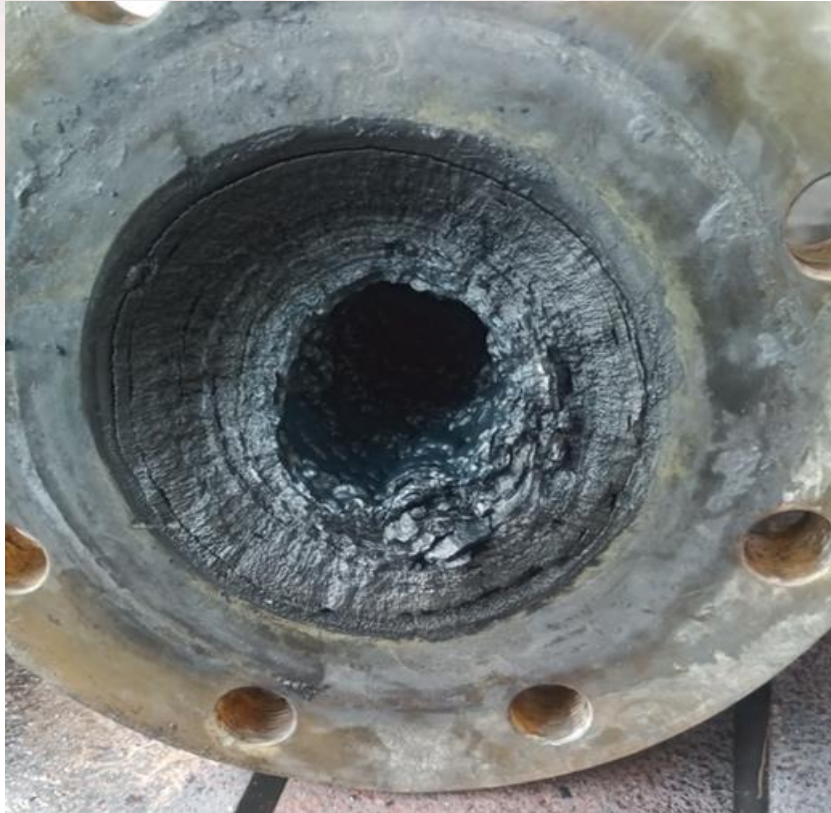
Quench tower circulation pipes blocking
