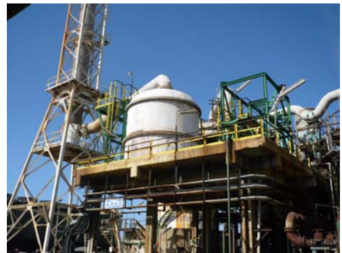
Wet Catalysis Plant filter vessel
