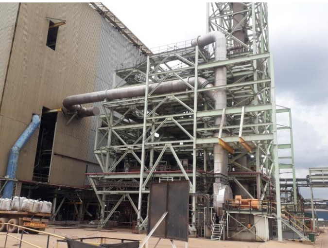
Kamoto Na-enhanced Lime Slurry Scrubber Installation
