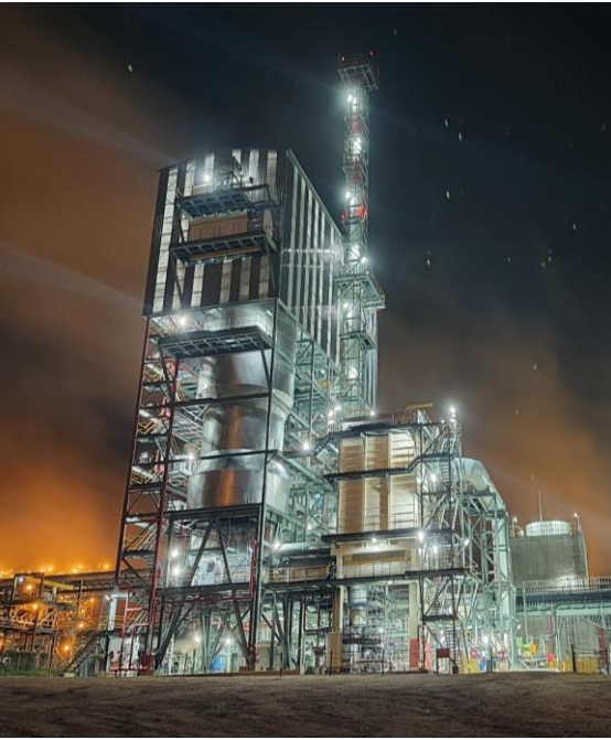
Anglo Platinum Polokwane Smelter WSA Plant
