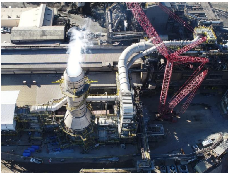
Freeport Miami Aisle \text{SO}_2 Scrubber During Construction
